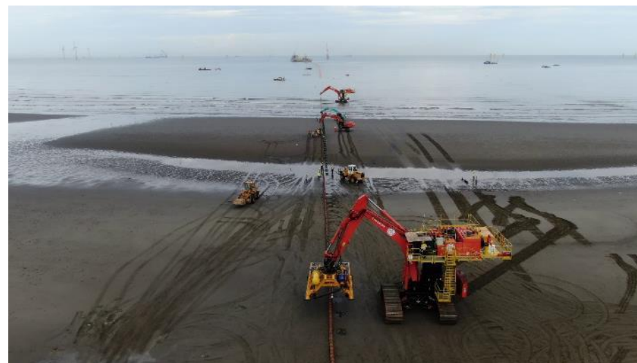
Figure 36 Offshore array cables installed at landfall. Image courtesy of Jan de Nul. All rights reserved.
