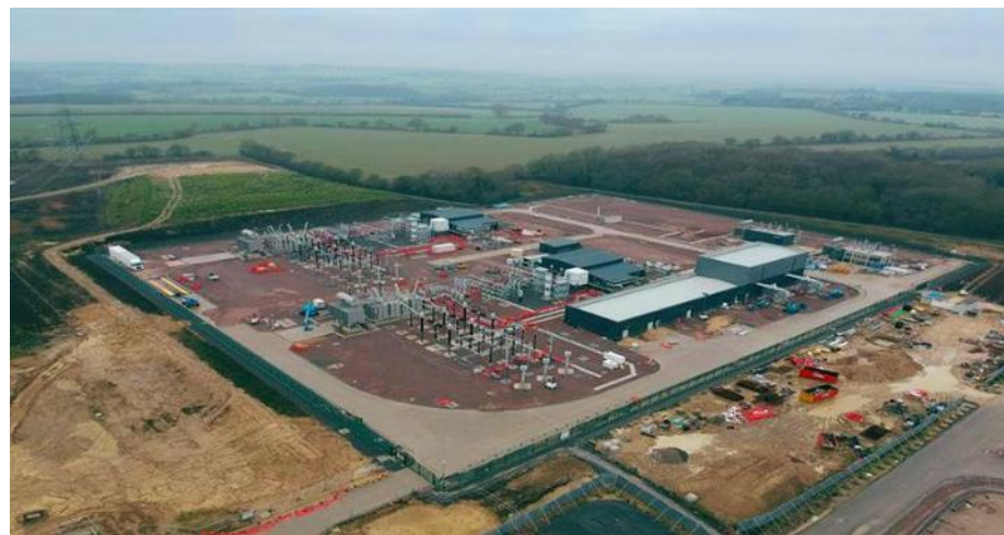
Figure 34 Onshore substation. Image courtesy of ScottishPower Renewables. All rights reserved.
