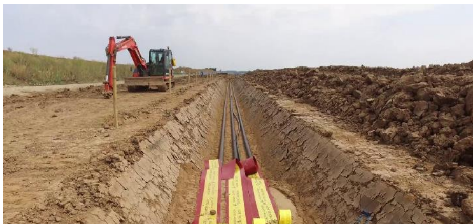
Figure 38 Onshore export cable trenching process. Image courtesy of Ørsted. All rights reserved.
