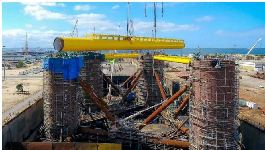
Figure 25 The final assembly of the primary structure of a steel semi-submersible floating substructure. Photo of the WindFloat Atlantic project courtesy of Principle Power/Ocean Winds.
