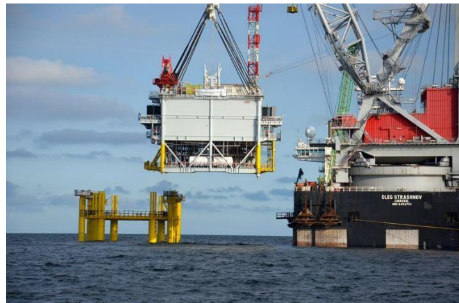
Figure 35 Topside structure of an offshore substation being lifted onto a jacket foundation. Image courtesy of ScottishPower Renewables. All rights reserved.
