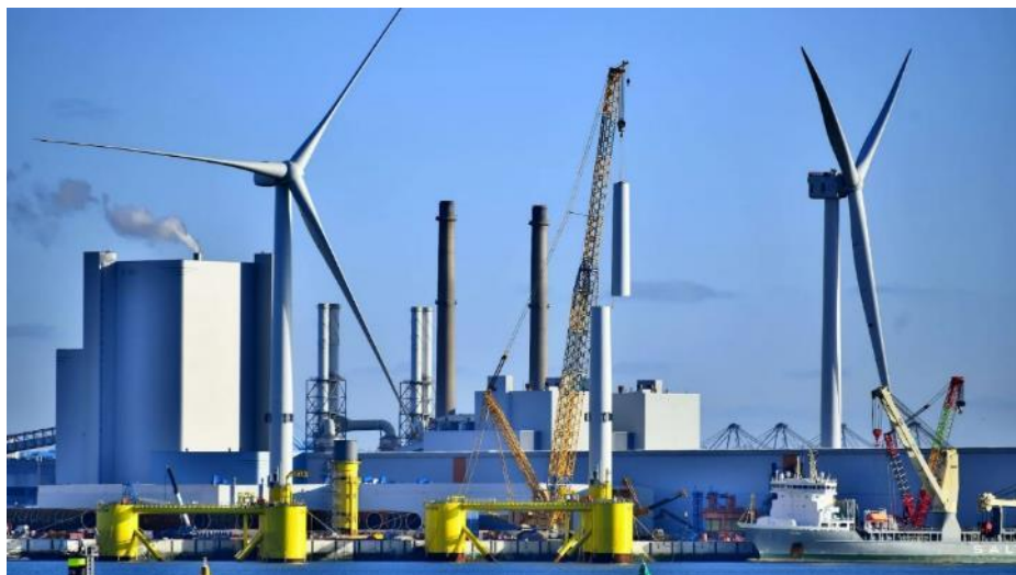
Figure 41 Floating offshore wind turbine final assembly taking place at port. Photo of the Kincardine Offshore Wind Farm project courtesy of Principle Power.
