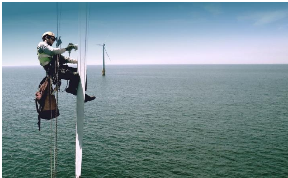
Figure 45 Blade inspection and minor repair being carried out by a rope-access technician. Image courtesy of Altitec. All rights reserved.
