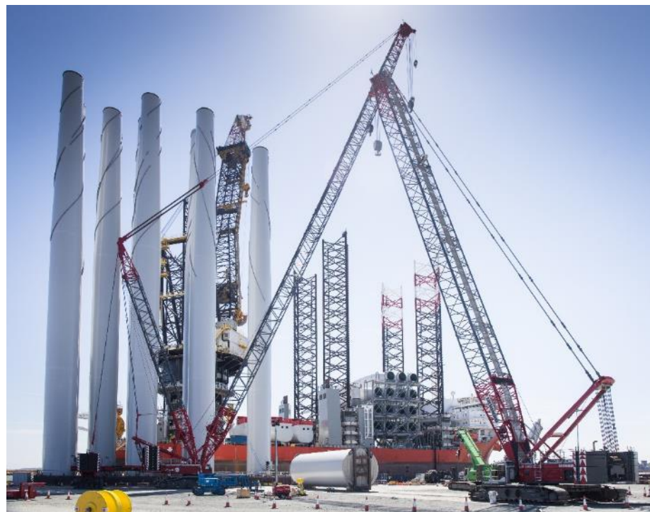
Figure 16 Offshore wind turbine towers being stored at the quayside of a port. Image courtesy of TMS. All rights reserved.
