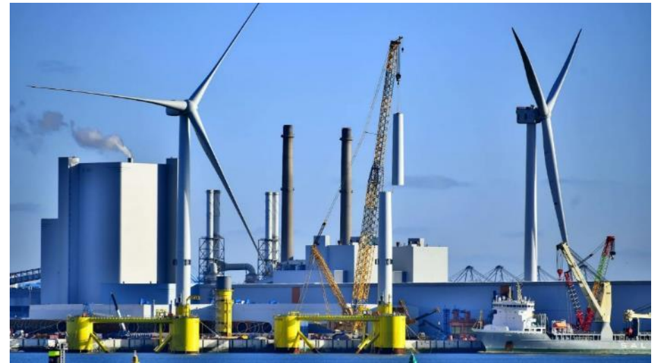
Figure 39 Floating offshore wind turbine final assembly taking place at port. Photo of the Kincardine Offshore Wind Farm project courtesy of Principle Power.
