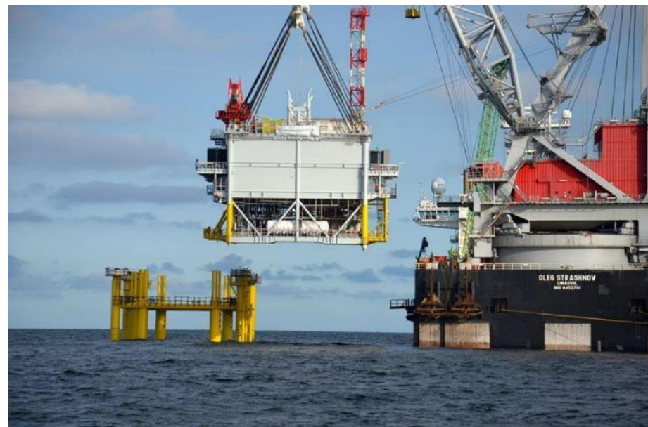
Figure 33 Topside structure of an offshore substation being lifted onto a jacket foundation. Image courtesy of ScottishPower Renewables. All rights reserved.
