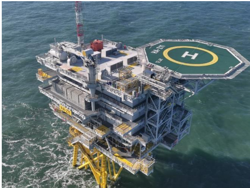
Figure 30 One of the fixed offshore substations used at the Hornsea One project. Image courtesy of Ørsted. All rights reserved.
