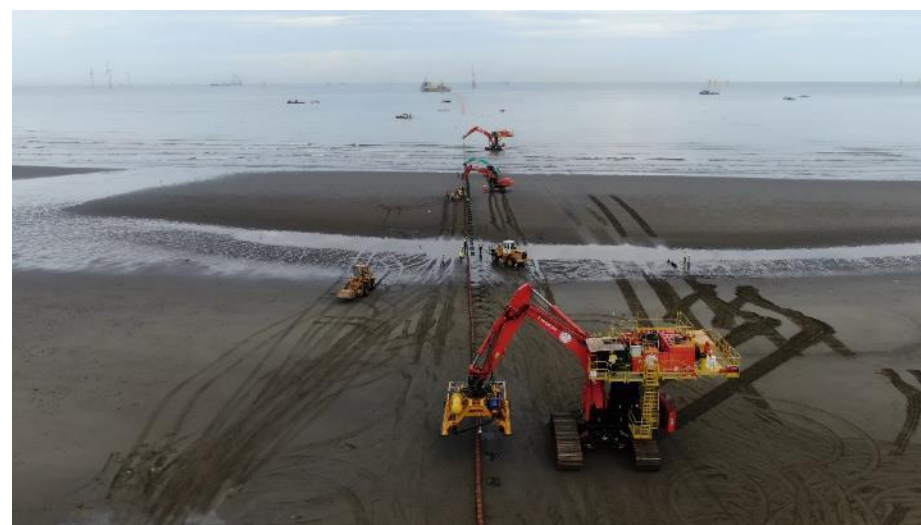
Figure 34 Offshore array cables installed at landfall. Image courtesy of Jan de Nul. All rights reserved.
