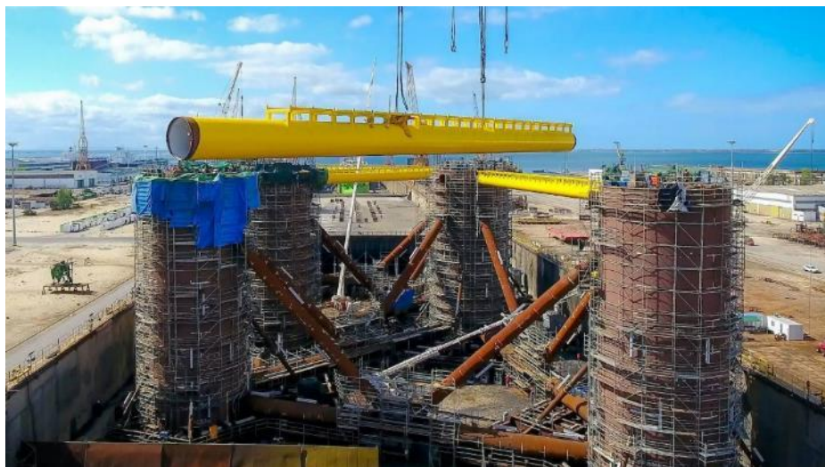
Figure 23 The final assembly of the primary structure of a steel semi-submersible floating substructure. Photo of the WindFloat Atlantic project courtesy of Principle Power/Ocean Winds.
