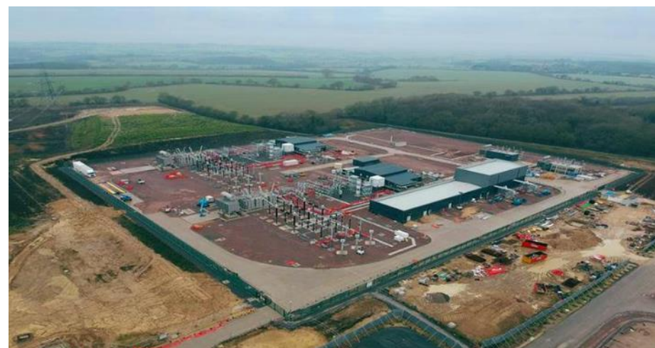
Figure 32 Onshore substation. Image courtesy of ScottishPower Renewables. All rights reserved.
