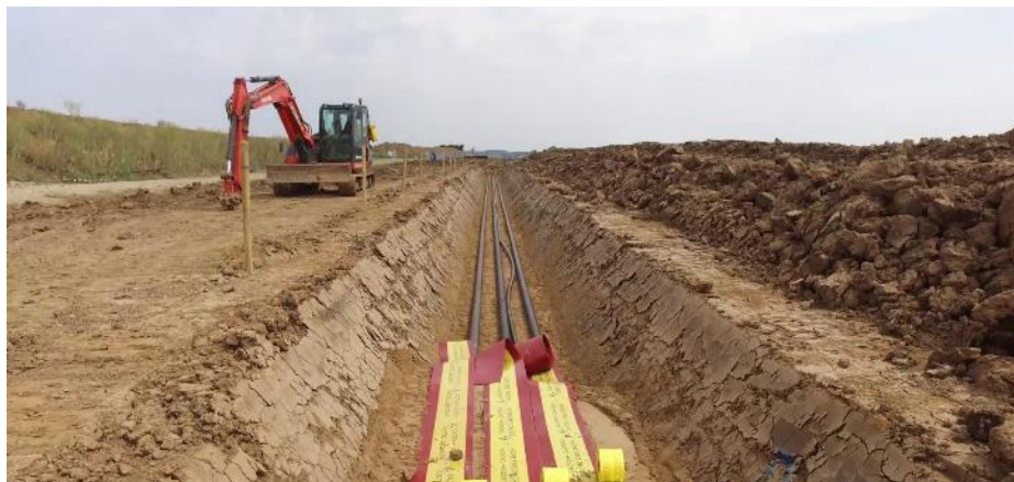
Figure 36 Onshore export cable trenching process. Image courtesy of Ørsted. All rights reserved.
