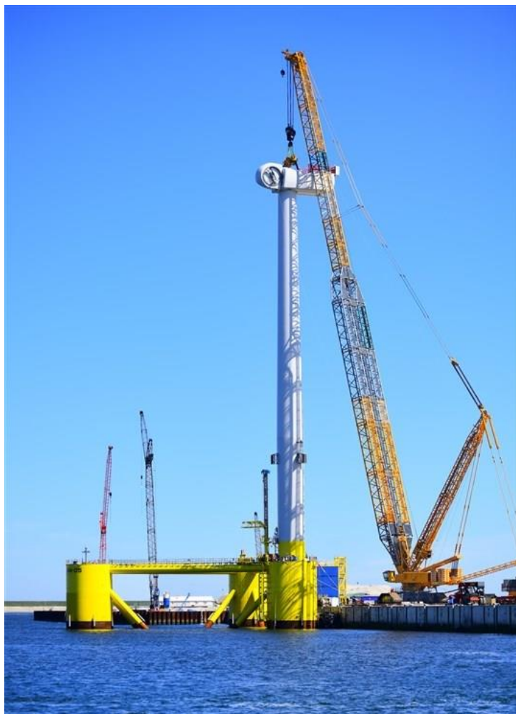
Figure 40 A landside crawler crane lifting a nacelle onto a floating substructure. Image courtesy of Port Pictures / Danny Cornelissen. All rights reserved.
