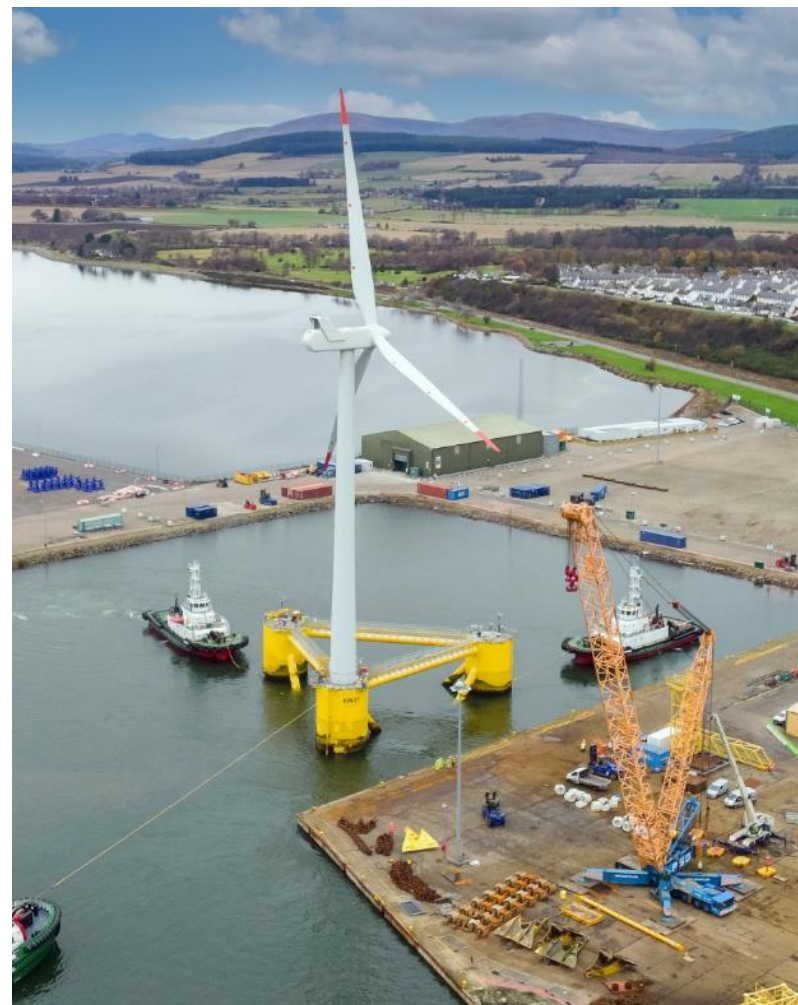
Figure 42 The Port of Cromarty Firth used as the construction port for part of the Kincardine project. Image courtesy of Port of Cromarty Firth. All rights reserved.
